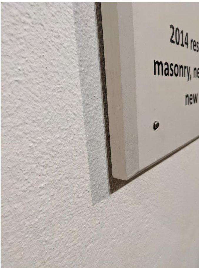
Air gap between wall and plaque
